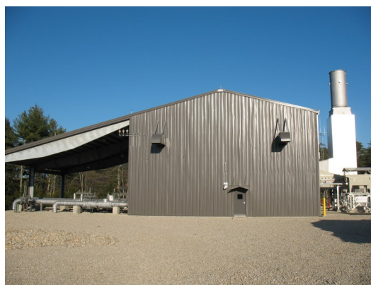
A compressor station on the TGP system in New Hampshire.
