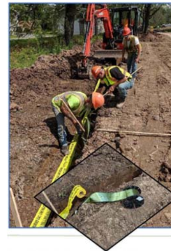
This photo illustrates field installations of MetGlas® in National Fuel Gas territory in Buffalo, NY in 2019 - part of a project to evaluate amorphous metal tape as a practical application for PE pipe location. Source: NYSEARCH
