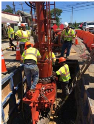
Photo: National Grid
