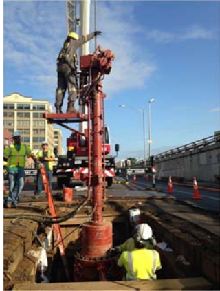
Photo: National Grid
