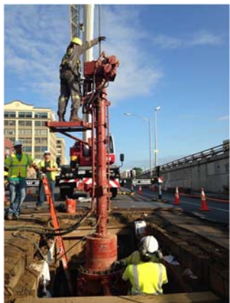
Photo: National Grid
