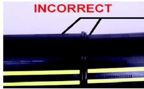
Improper "High-Low" alignment
