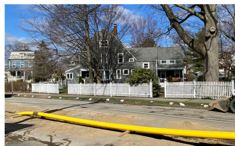
A natural gas distribution line being upgraded and about to be installed, outside Boston, in spring 2021.
