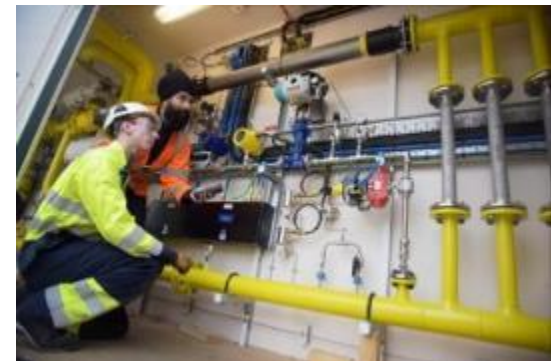
100 v% methane versus 28 v/v% hydrogen/methane – “HyDeploy: The UK’s First Hydrogen Blending Deployment Project”
