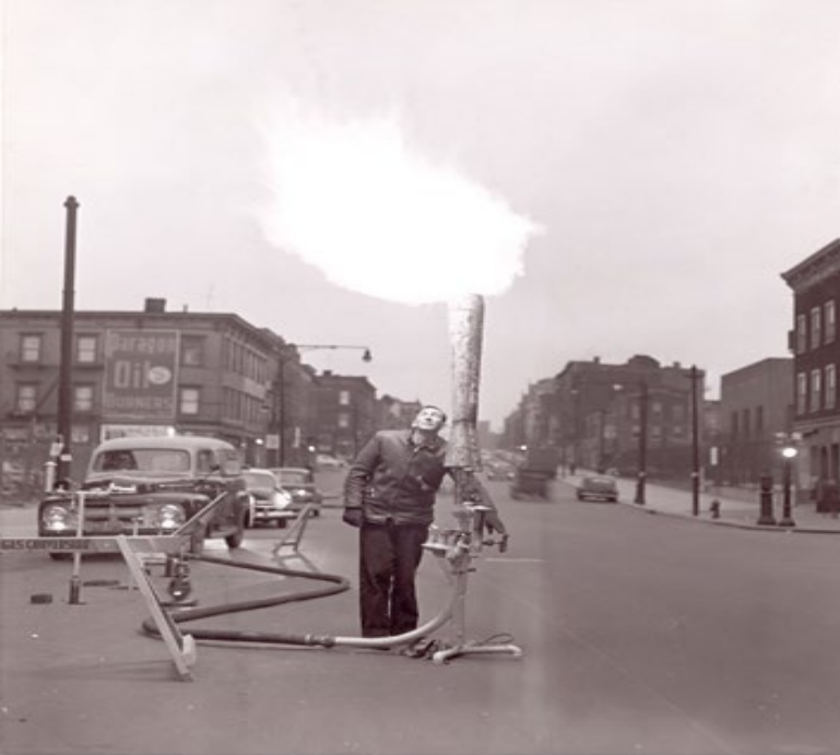
A purge burner igniting manufactured gas being replaced in a main by natural gas during the 'great conversion' in 1952
