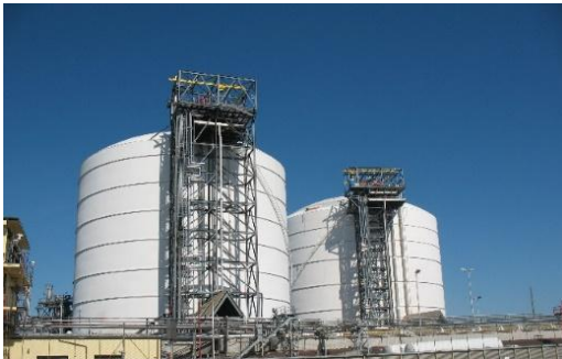
Everett LNG facility, part of Exelon (Constellation)
