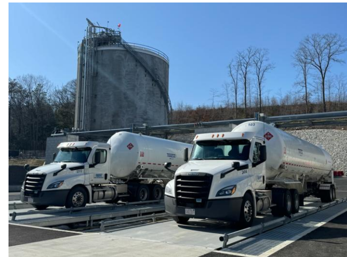
Northeast Energy Center
