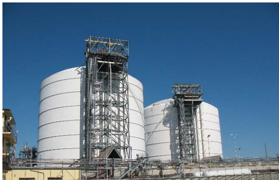
Everett LNG facility, part of Exelon (Constellation)
