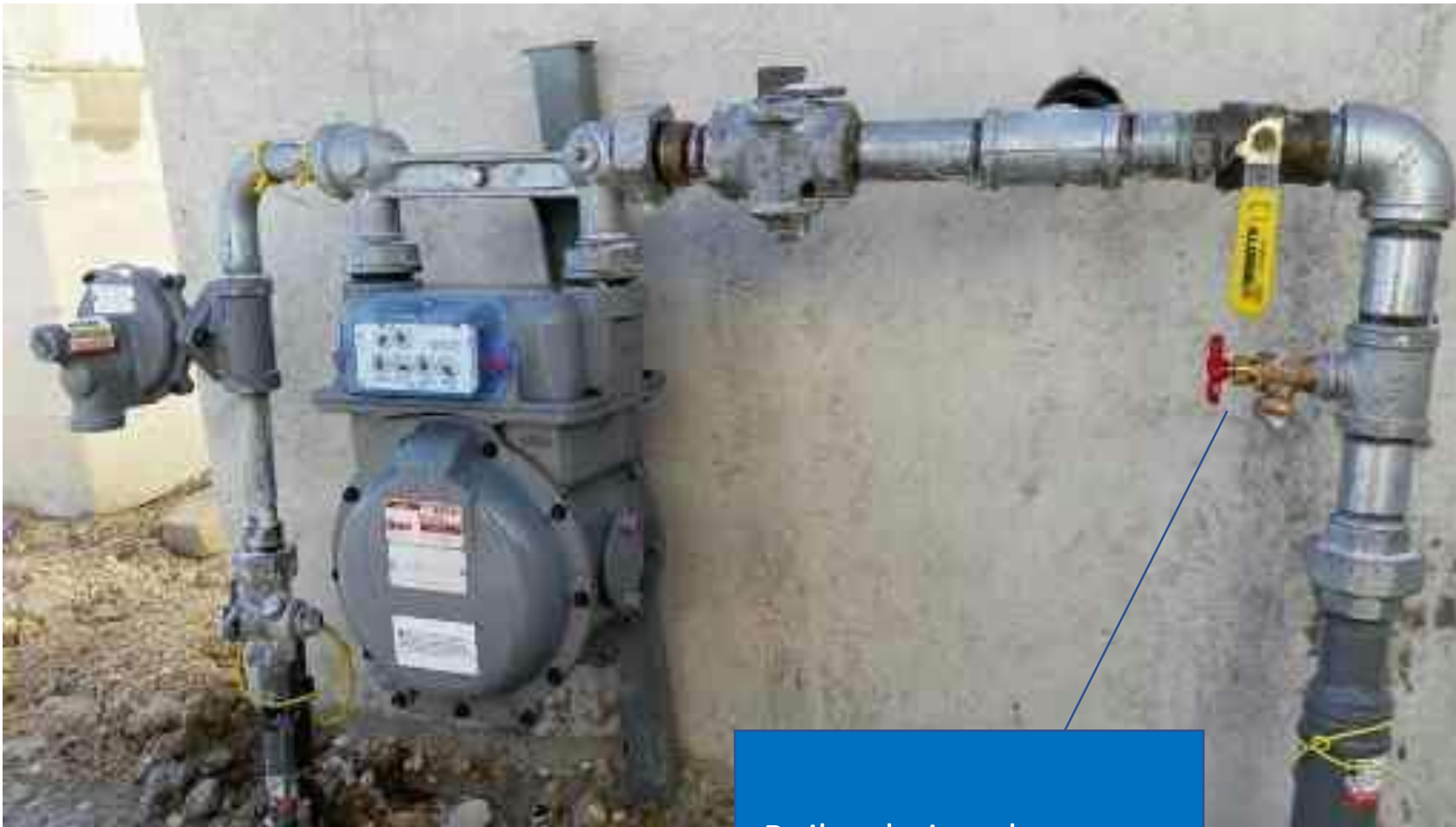
Boiler drain valve on gas piping (NG)
